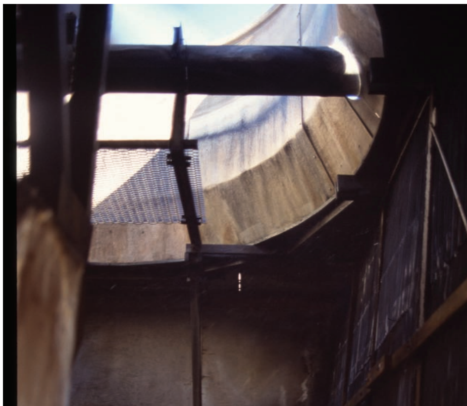
Open to the environment, cooling towers are highly efficient collectors of particles and debris.
